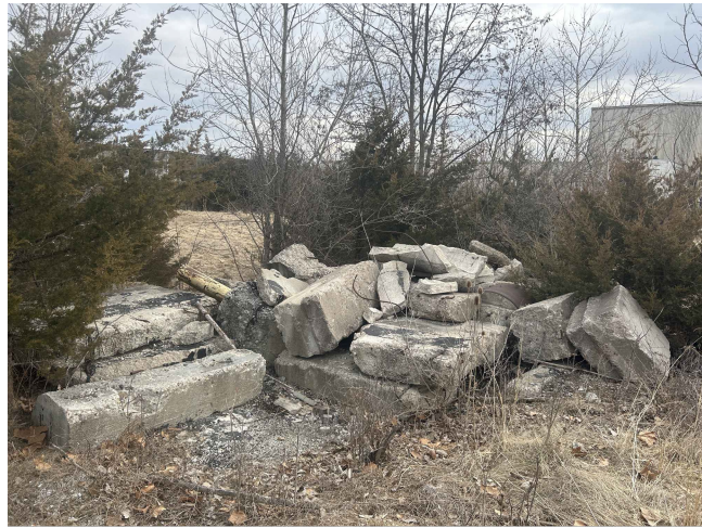
CONCRETE DEBRIS TO BE REMOVED
