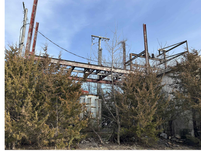
DEFUNCT EQUIPMENT TO BE REMOVED
