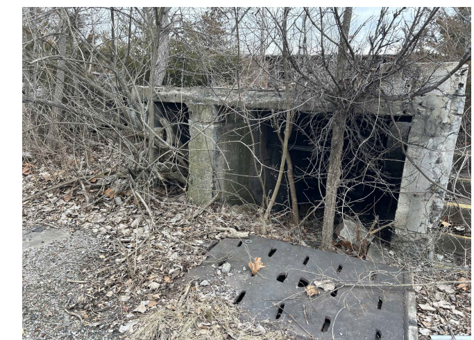
STORMWATER DRAIN TO BE COVERED
