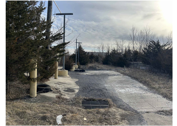
STORMWATER DRAIN TO BE COVERED POLES AND CONCRETE TO BE REMOVED
