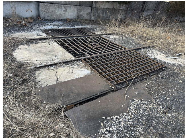
STORMWATER DRAIN TO BE COVERED
