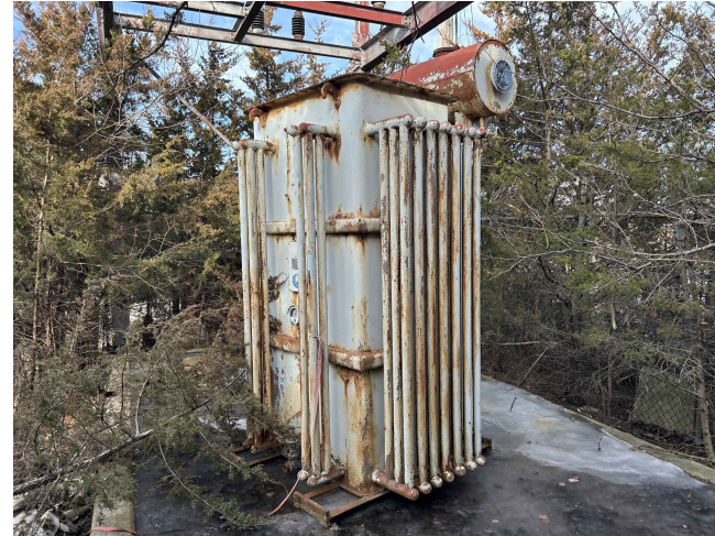
DEFUNCT TRANSFORMER TO BE REMOVED
