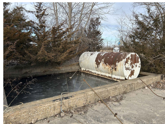
STORAGE TANK TO BE REMOVED
